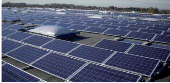
Solar installation in Derching/Germany, Photo: abakus solar AG
